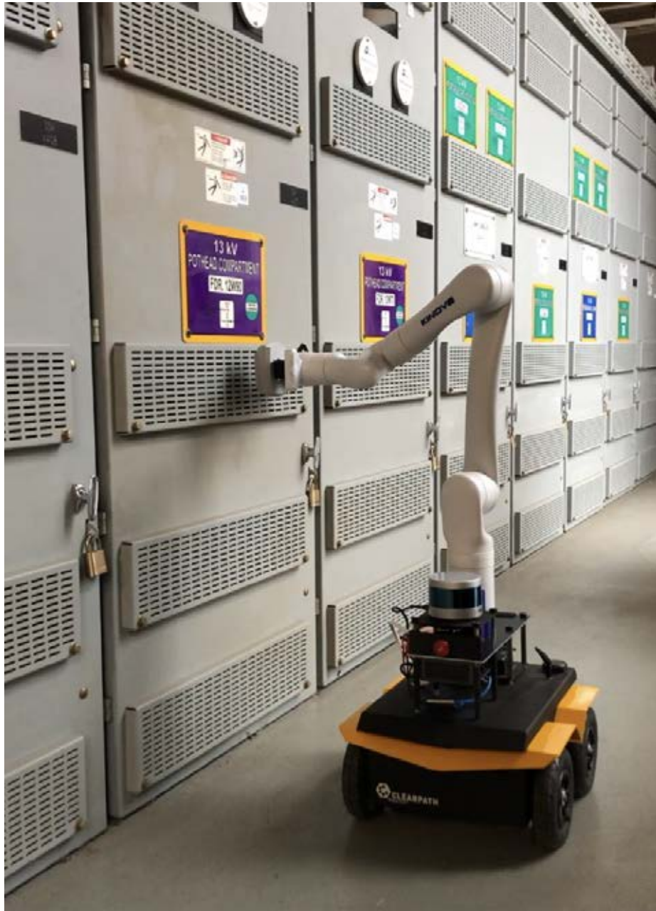
Figure 7.1: Mobile Manipulation in a Substation
